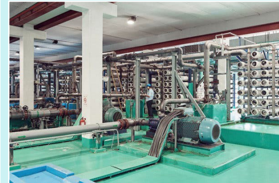
The reverse osmosis membrane tubes and electric water pressure pumps at Saudi Arabia's SAWACO Desalination Plant in Jeddah. (Source: New York Times)
